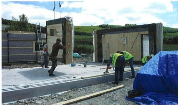
Second wall being placed with (in foreground) sole being fixed Greenhus Ltd.
